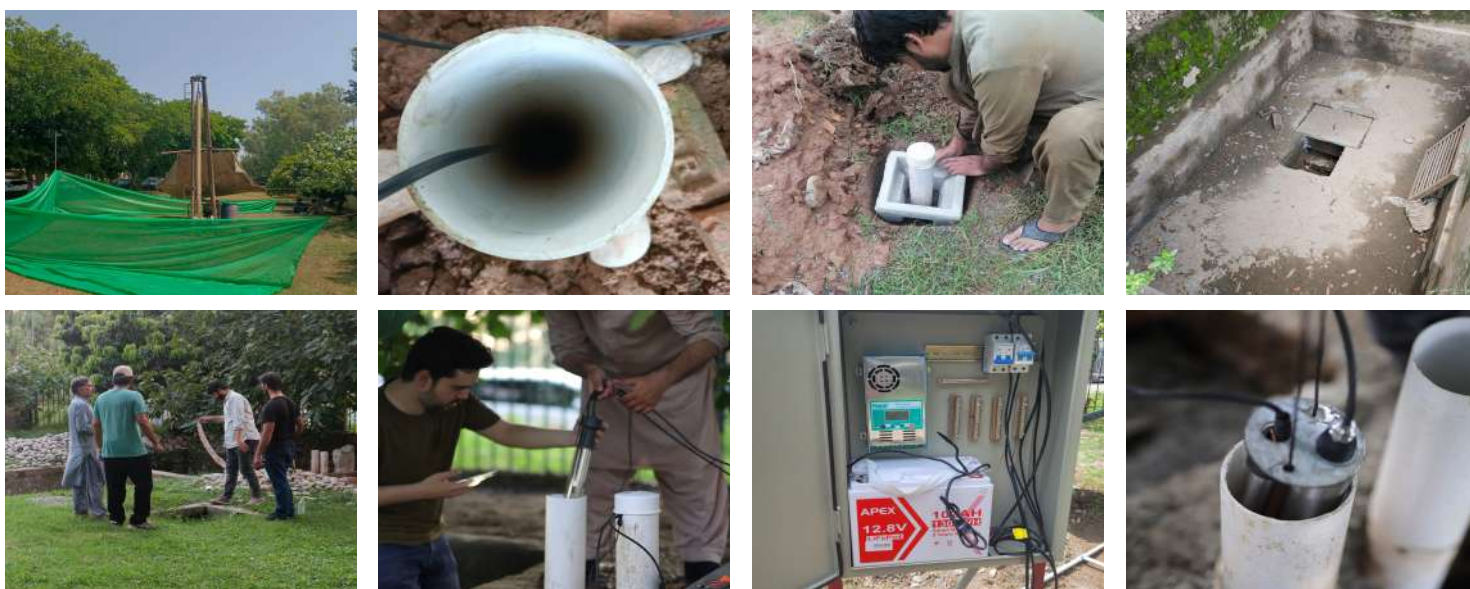
Figure 5.1: Snapshots of recharge well remodeling and upgrades undertaken to enable sensor installation, IoT-based monitoring and dashboard integration.
